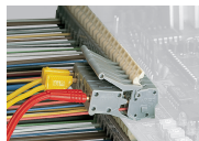
Testing with test plug modules.
