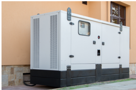
Engine / Generator starting
