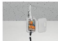
Pendant light connection in a suspended ceiling
