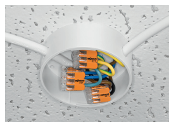
Lighting distribution in a ceiling canopy
