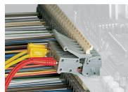
Testing with test plug modules.
