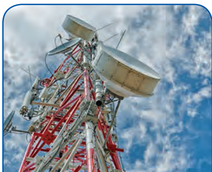
Telecom -Data Infrastructure
