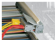
Testing with test plug modules.
