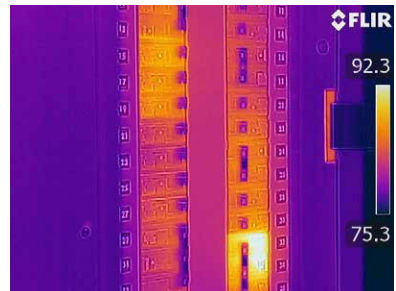
Overheating fuse in electrical panel
