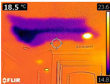
HVAC condensate overflow soaks a ceiling
