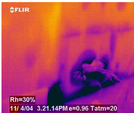
Moisture intrusion around electrical circuit
