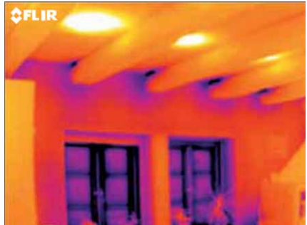
The thermal image shows thermal bridges between the roof beams and adjacent walls
