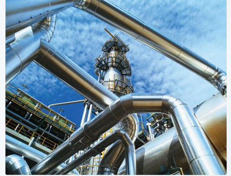
Chemical, Oil and Gas
